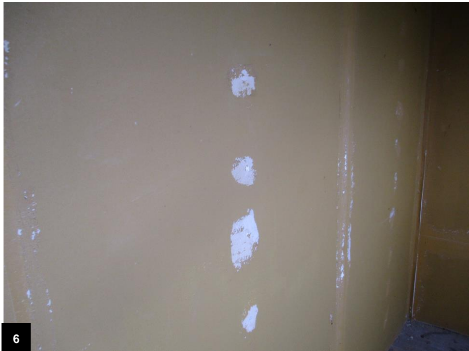
Sample 20 – Mustard Yellow Wall Paint – 3 rd Floor Stairway – 1088 Murphy Avenue 8.75 wt% Pb
