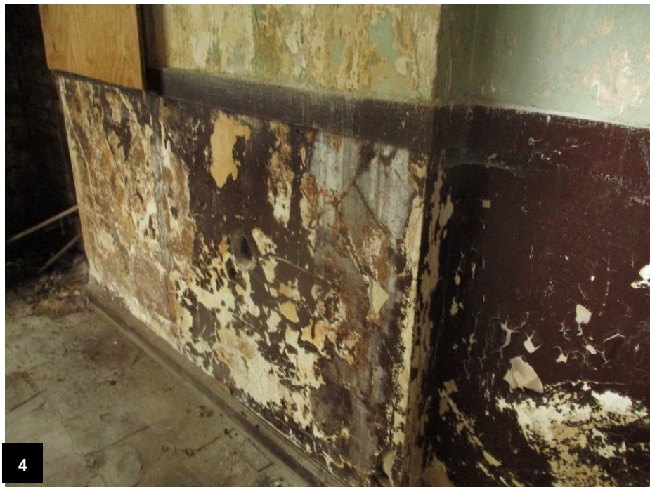
Sample 17 – Brown Wall Paint – North Wall 2 nd Floor – 1088 Murphy Avenue 1.42 wt% Pb
