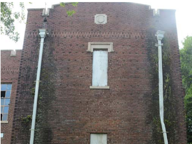
Figure 49. Environmental and biological discoloration near downspouts.
