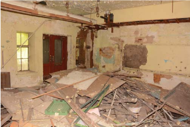
Figure 42. Debris piled up in a basement room.
