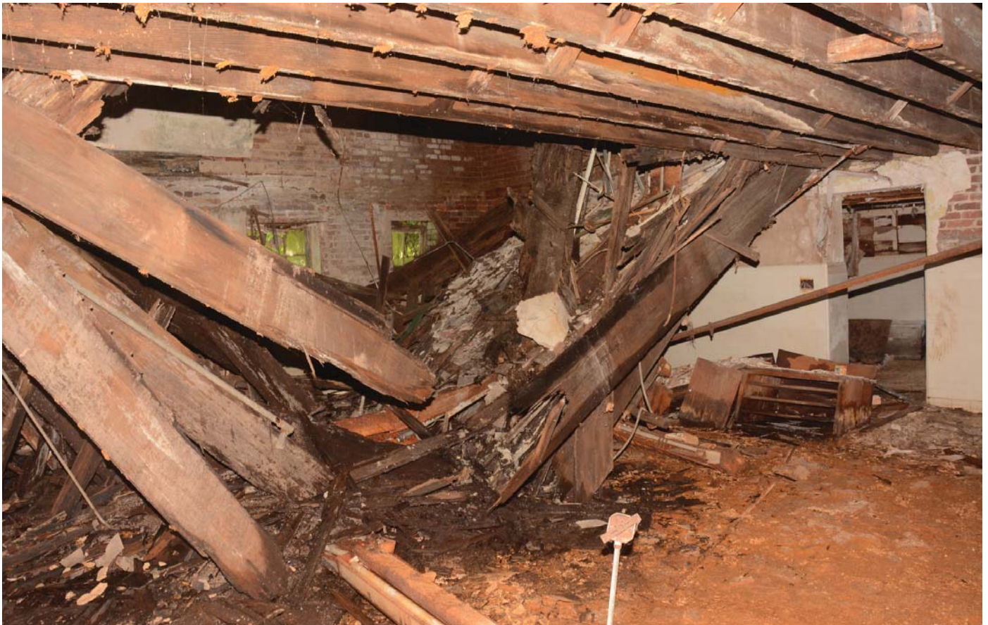
Figure 46. Unfortunately typical condition of the wood joists.
