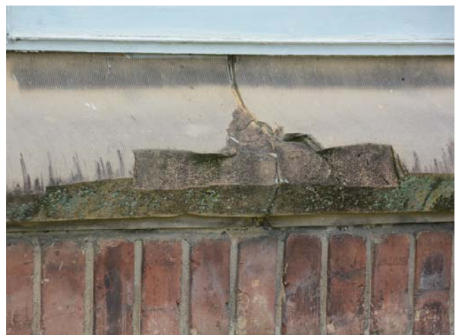
Figure 52. Typical terracotta damage.
