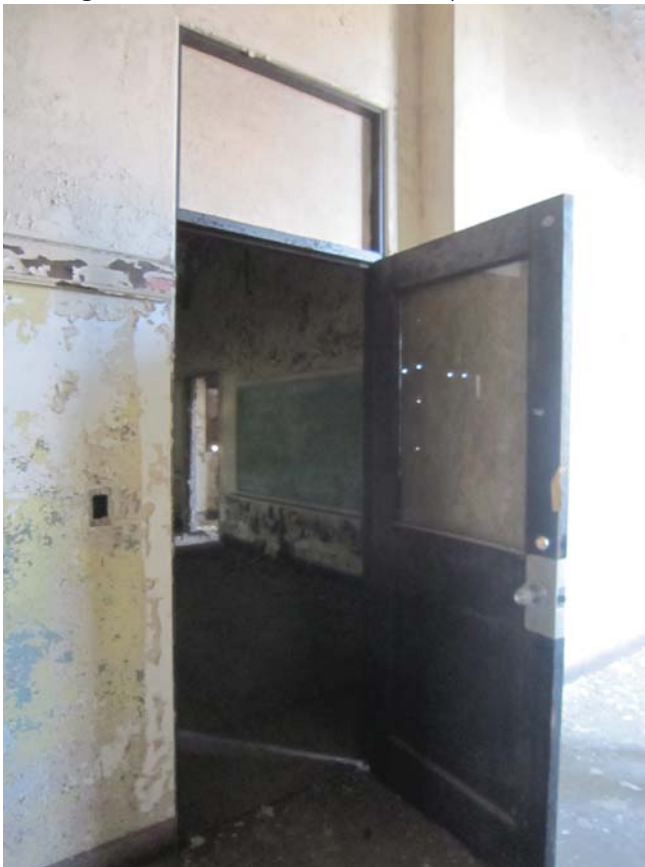
Figure 79. Extant Type B door with boarded up transom lite.
