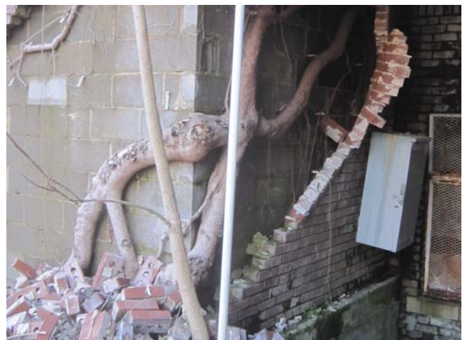
Figure 50. Non-Historic concrete block addition with tree roots.
