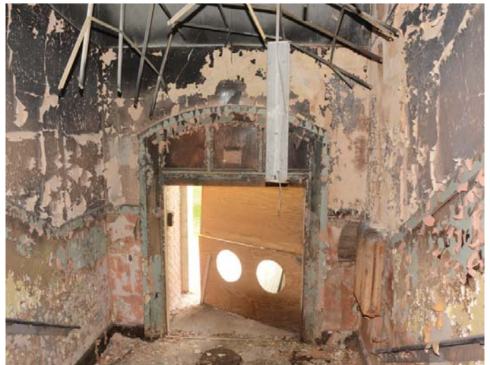
Figure 77. Missing doors as west entrance to the building.
