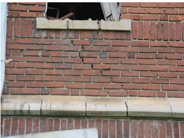
Figure 51. Isolated step cracking on west elevation.
