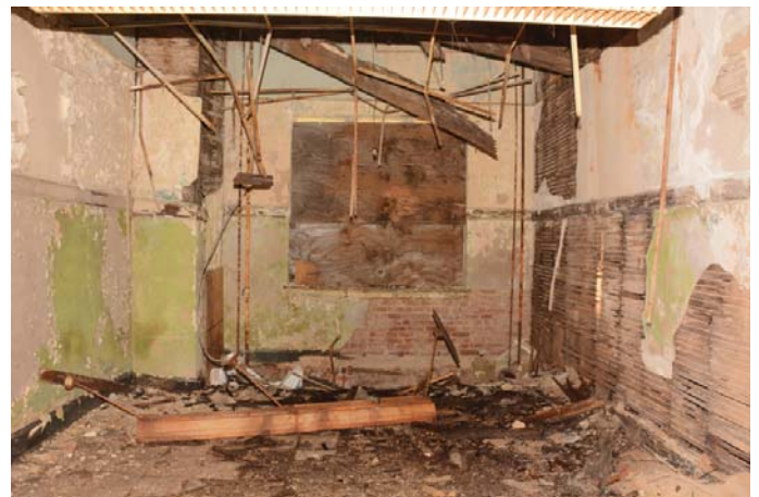
Figure 22. A more typical wall and plaster condition found in the 1911 section.
