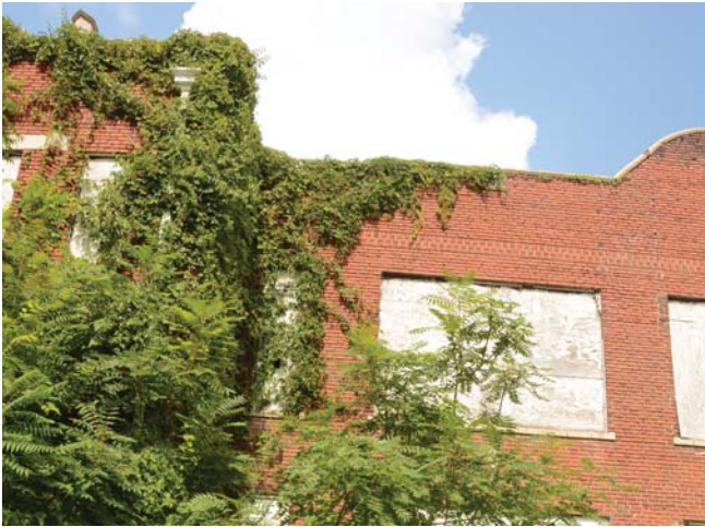
Figure 47. Vegetation growth on exterior walls.
