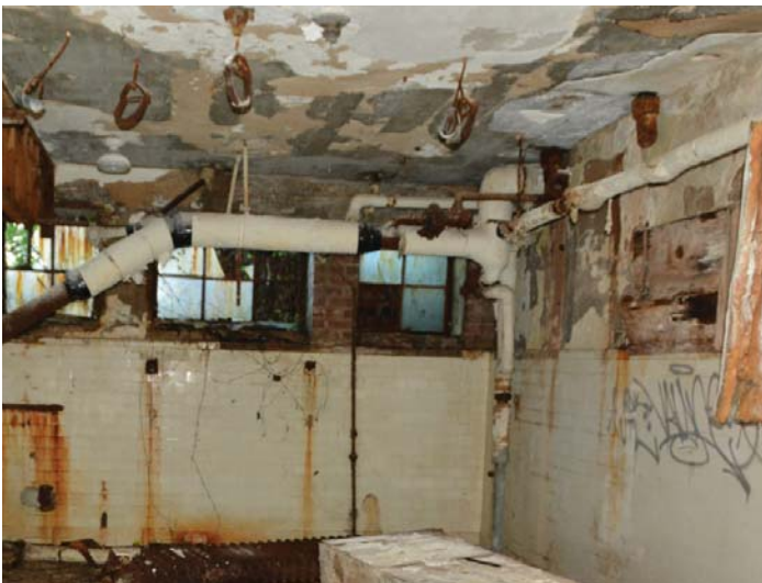
Figure 83. Old Plumbing in Basement
