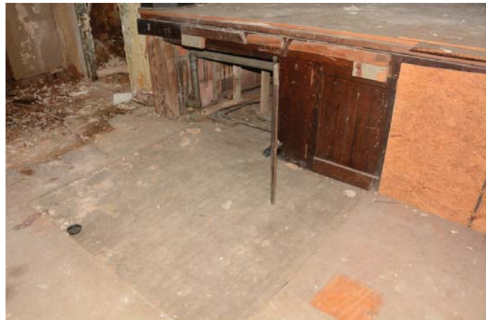
Figure 60. Exposed wood flooring in the auditorium.
