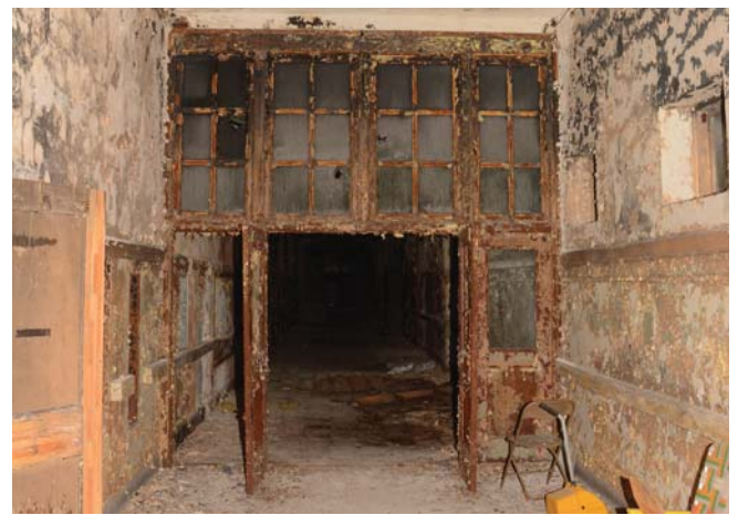
Figure 35. Steel door and window corridor partitions at first floor. There is a non-historic basement corridor partition with six-lite double-doors framed in a flat plaster wall.
