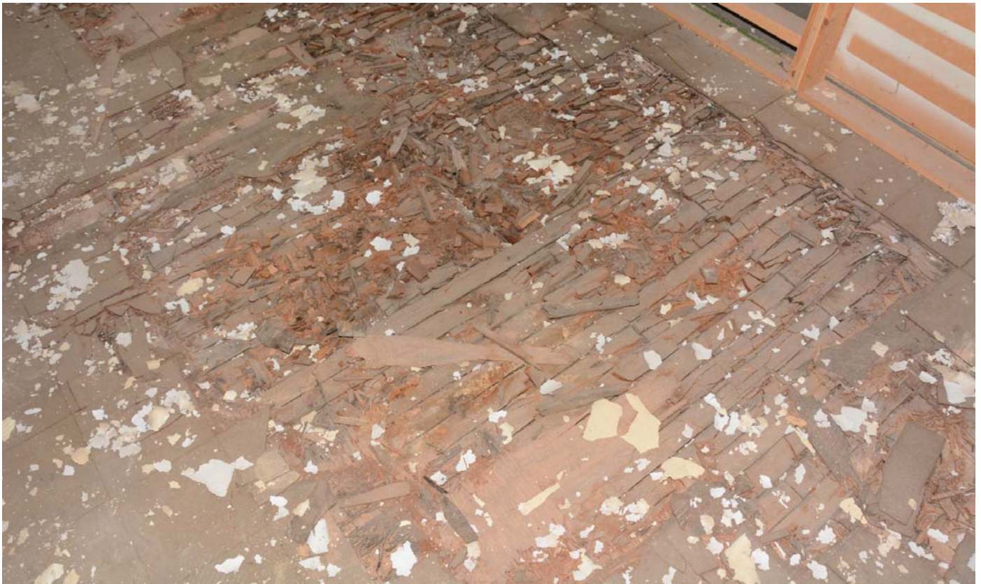
Figure 23. Detail of flooring showing highly deteriorated tongue and groove wood flooring that was below plywood, 9x9 VAT, and 12x12 resilient tile.
