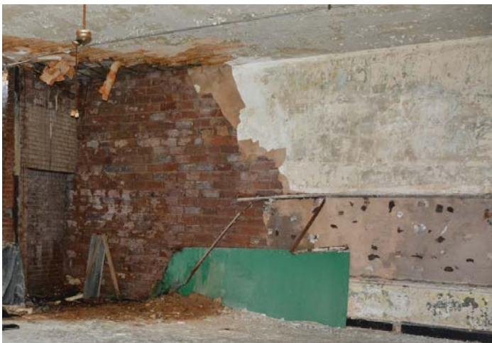
Figure 58. Classroom wall showing failed plaster next to stable plaster. A vertical joint will be cut at the stable plaster.
