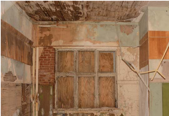
Figure 67. Failed plaster on wood lath ceiling above an intact wood window frame.
