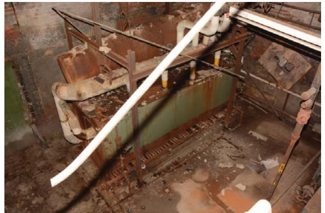
Figure 43. Some standing water was observed in the mechanical sub-basement.
