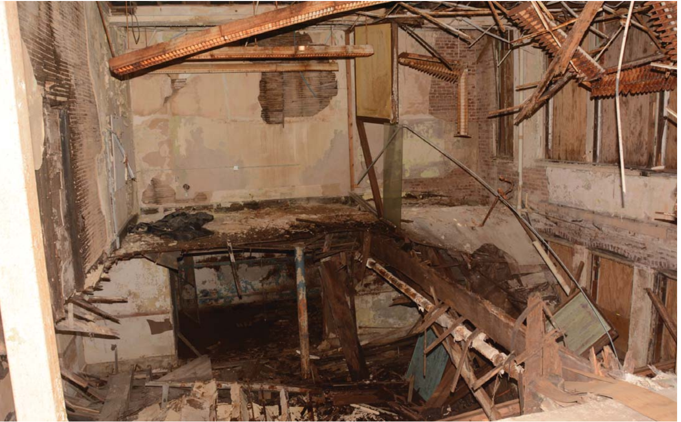
Figure 45. Wood Framing structural failure, Image also shows supplemental steel beam and column.
