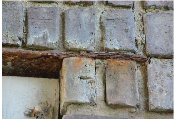
Figure 68. One of the few rusted window lintels that may need to be replaced.
