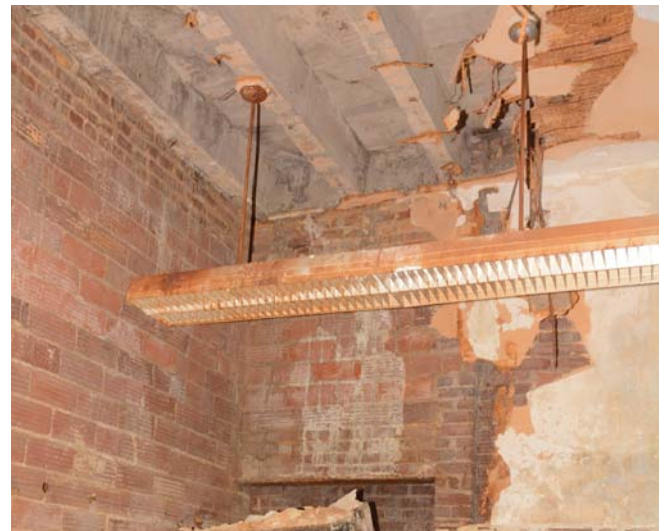
Figure 85. Obsolete Fluorescent lighting.
