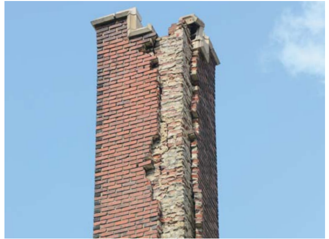
Figure 48. Brick Chimney showing failure of face brick.
