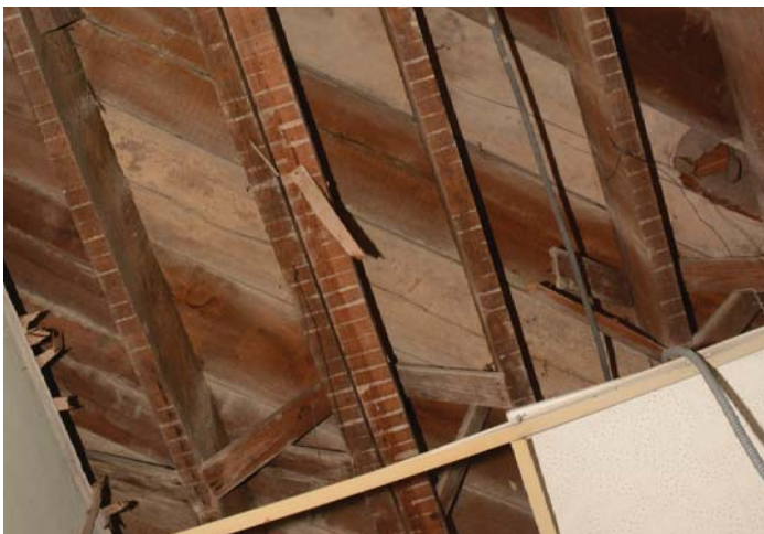
Figure 66. Removed plaster ceiling on wood lath above a non-historic suspended grid ceiling.
