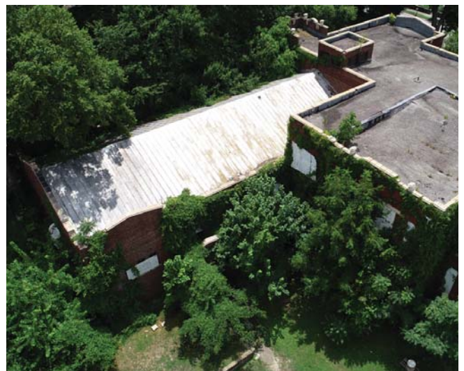
Figure 11. View of Auditorium roof with portions of the south wing and main building to the right.
