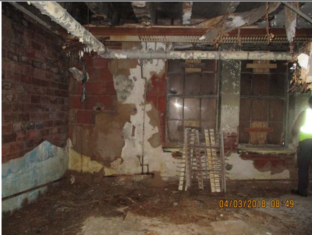
Terracotta brick foundation wall with minor damage that can be repaired.
