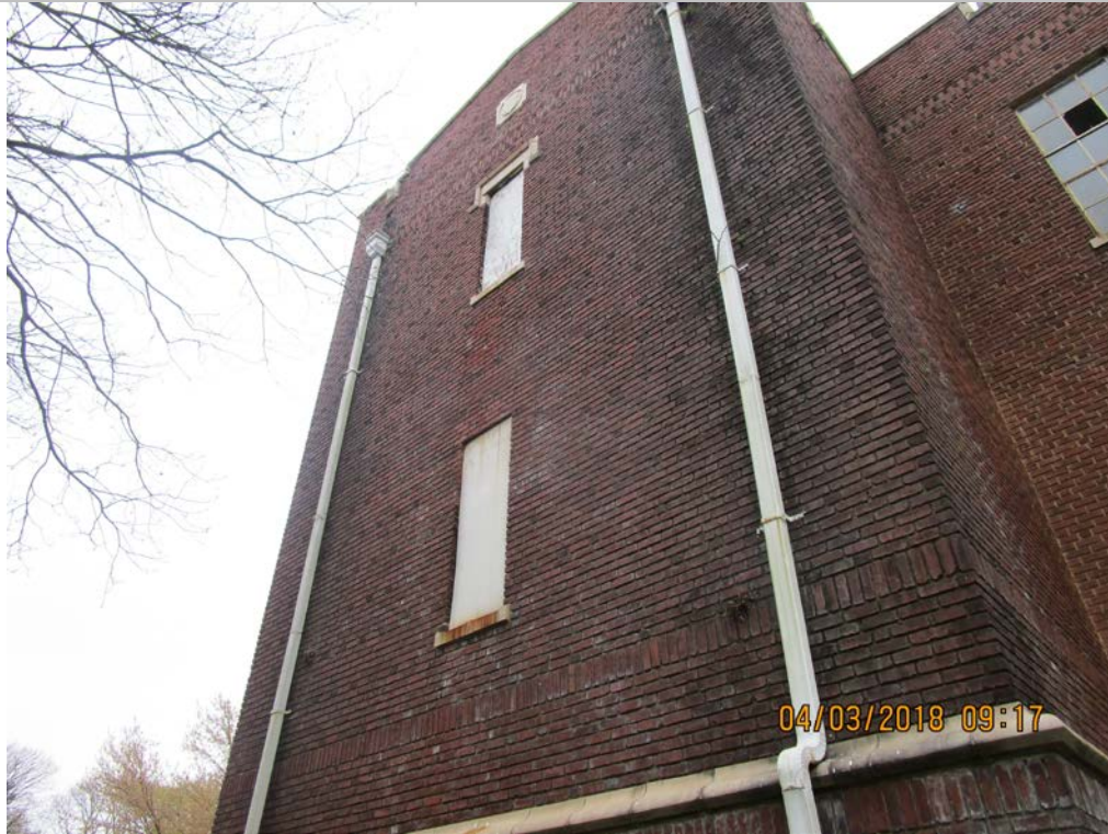
Exterior brick distress – water staining.
