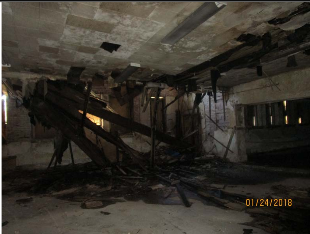
Part of the structure has collapsed.
