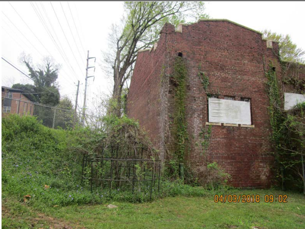
Exterior brick distress - cracking.
