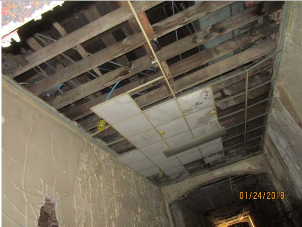
Wood floor framing deteriorated.
