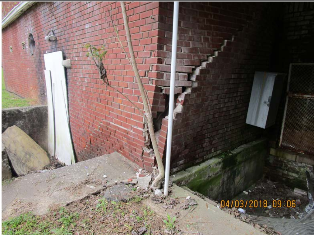
Exterior brick distress – cracking and collapse at attached storage.
