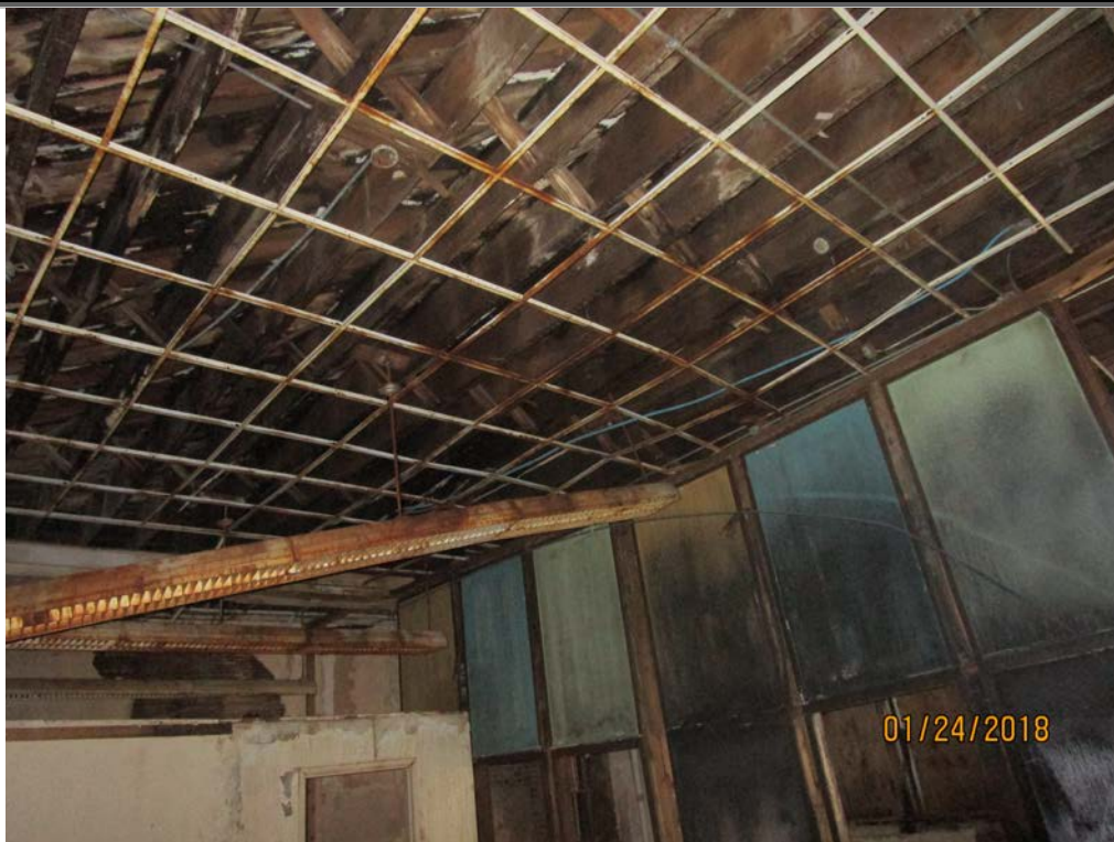
Wood floor framing deteriorated.
