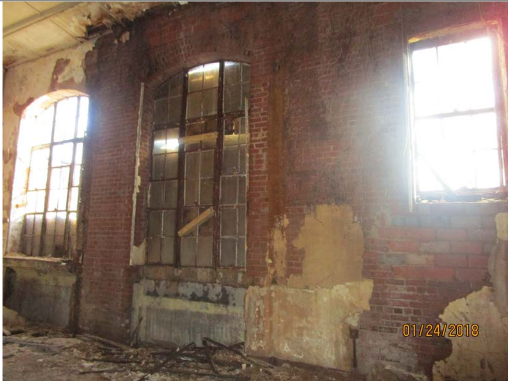
Vegetation growing through building envelope.
