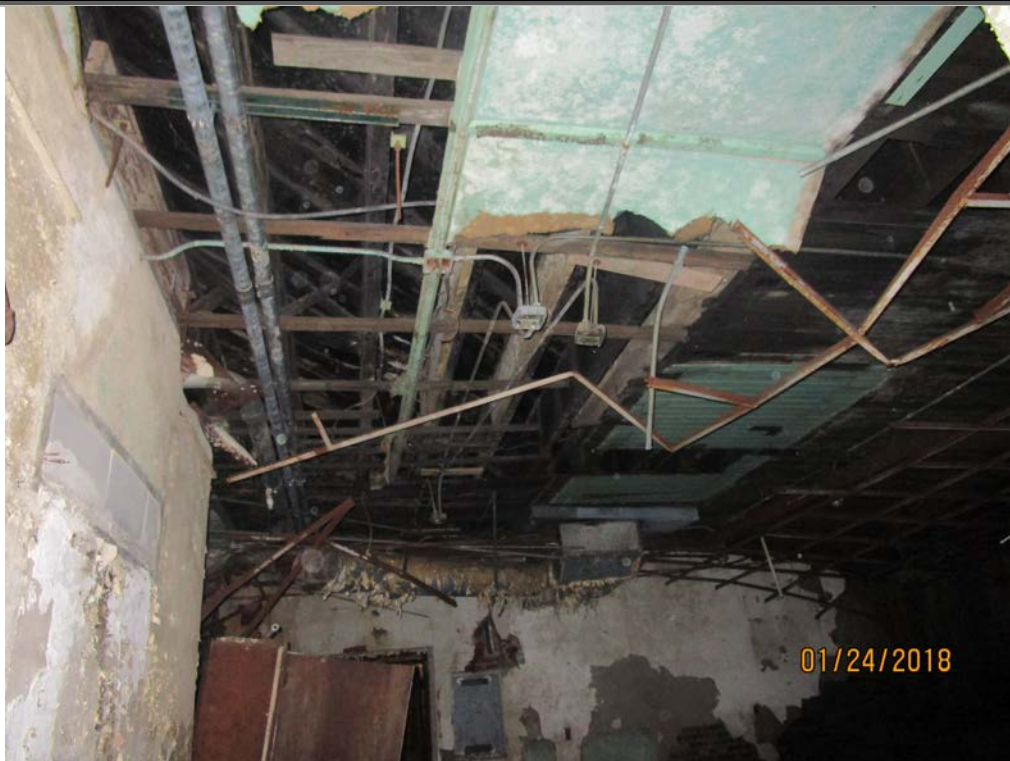
Wood floor framing deteriorated.
