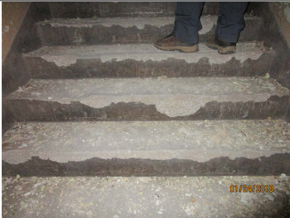
Some damage to concrete stairs that can be repaired.
