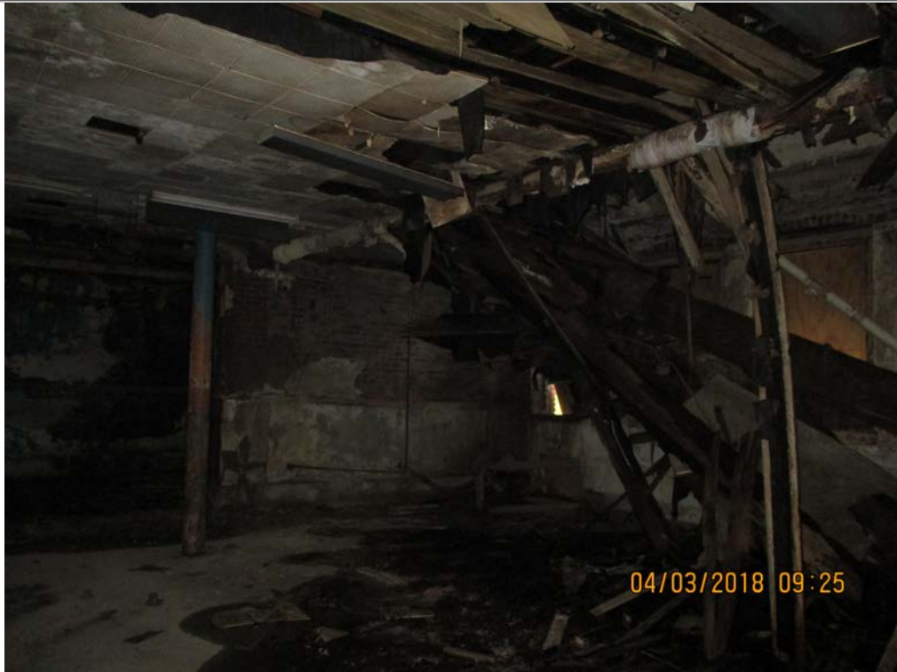
Wood floor framing deteriorated and collapsed.
