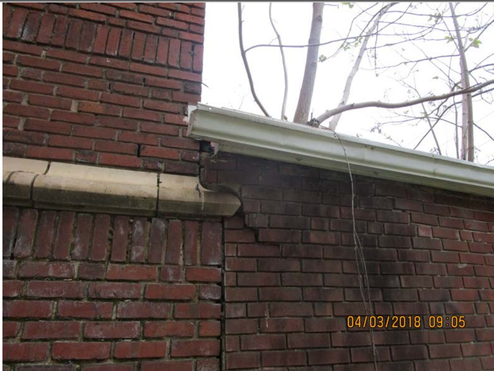
Exterior brick distress - cracking.
