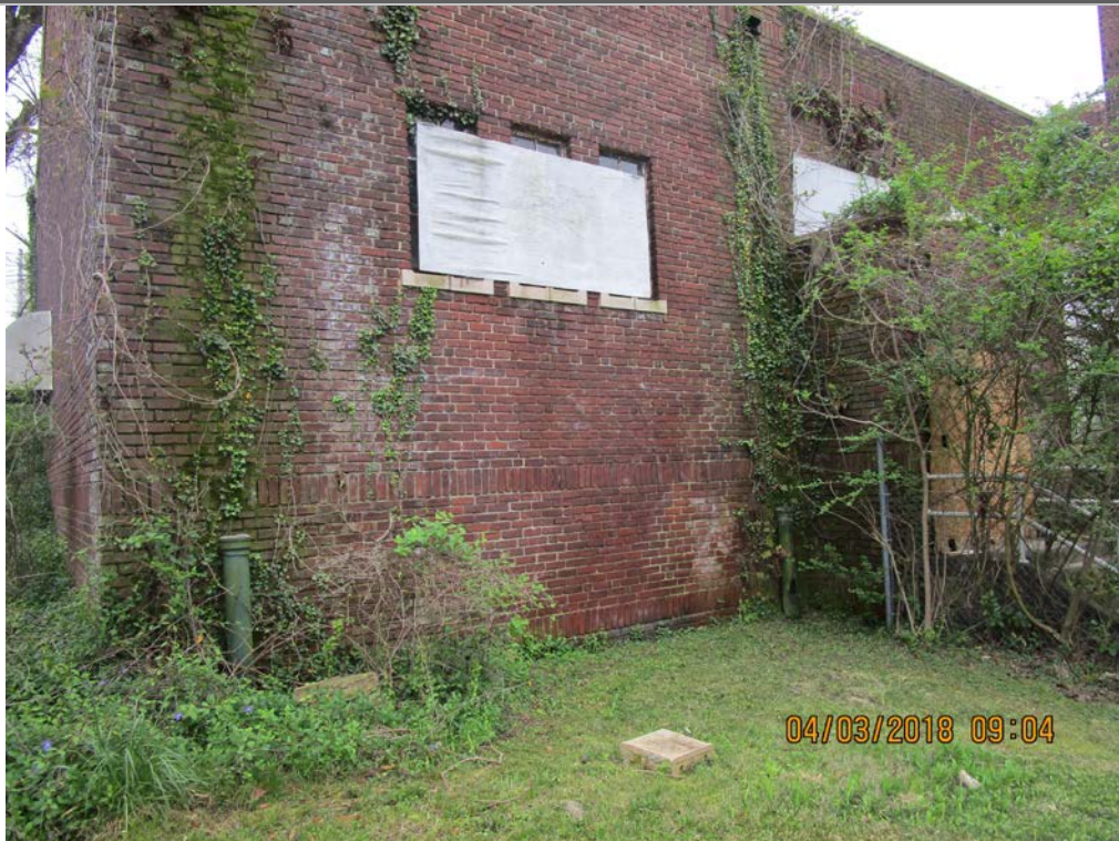
Exterior brick distress – water staining.
