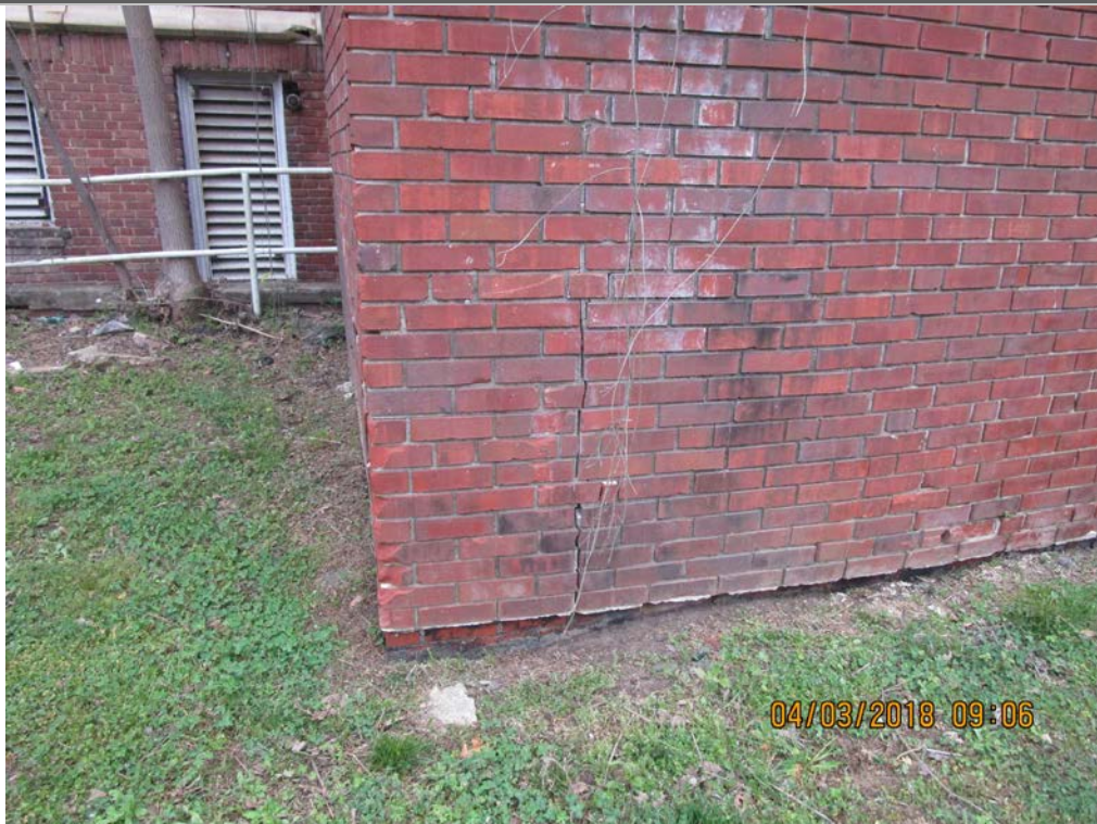
Exterior brick distress - cracking.
