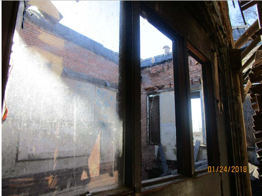
Part of the structure has collapsed.
