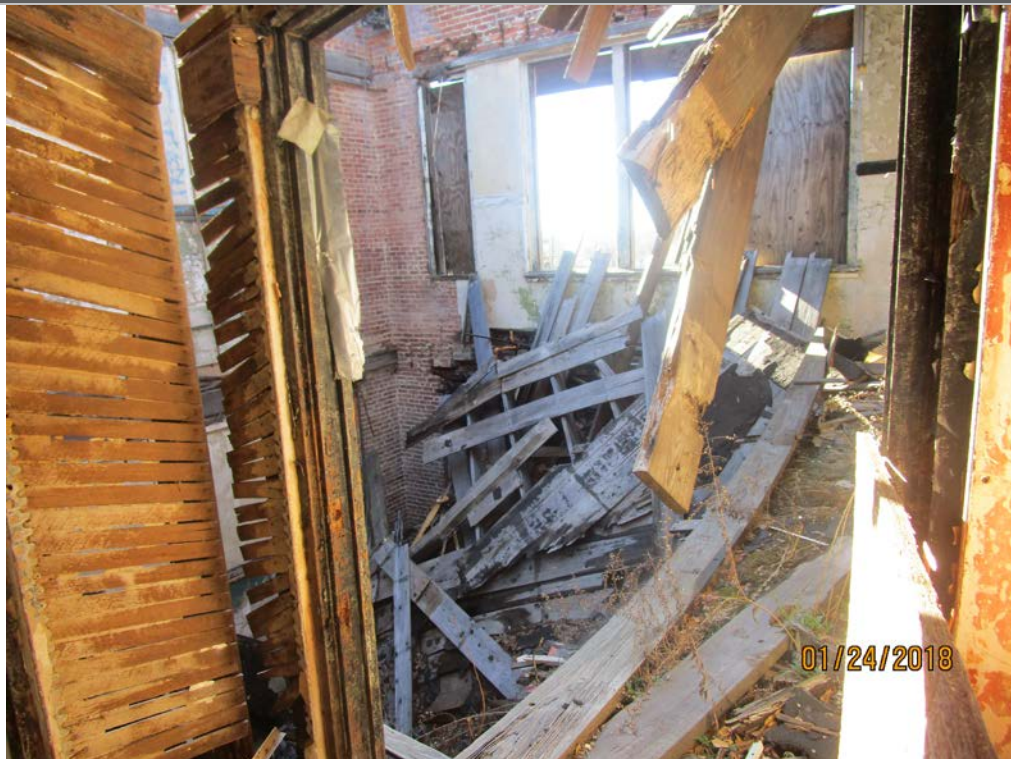
Part of the structure has collapsed.
