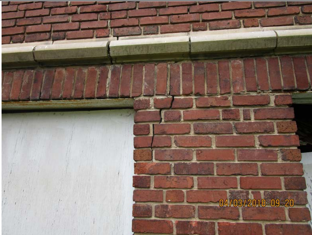
Exterior brick distress - cracking.
