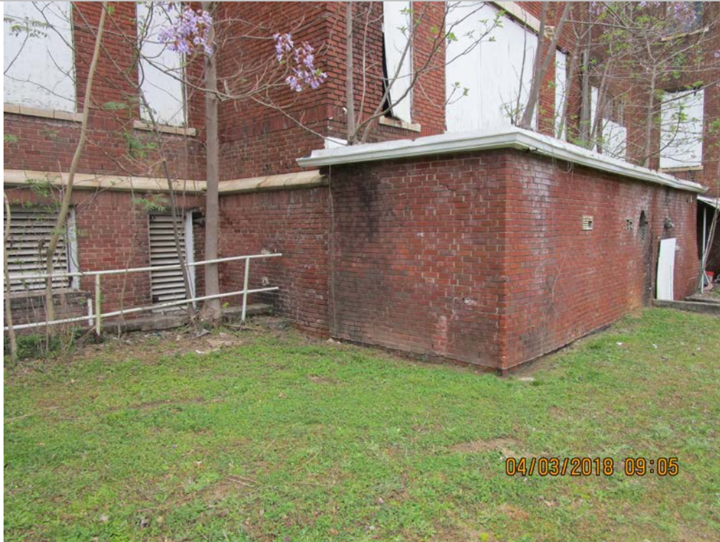
Vegetation growing on top of roof.
