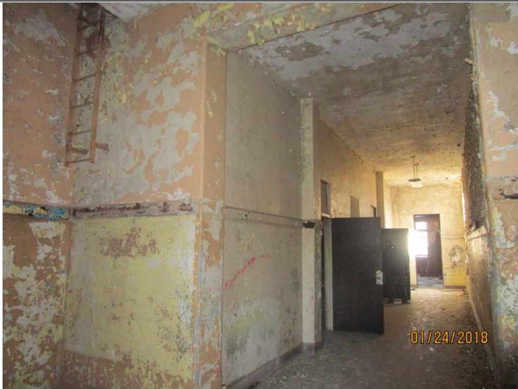
Roof system of left and right wing additions covered with plaster – further evaluation needed.
