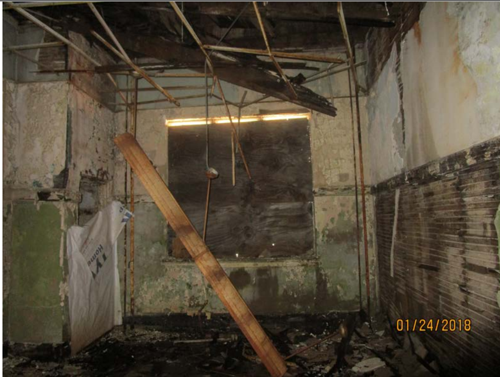
Part of the structure has collapsed.
