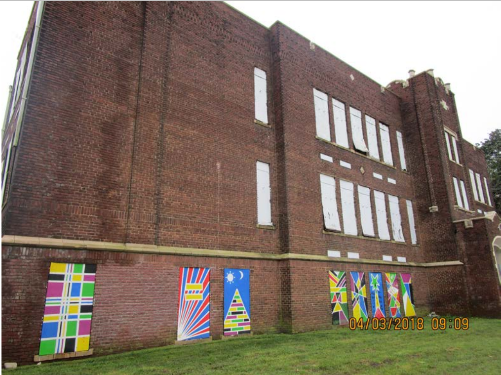
Exterior brick distress – water staining.
