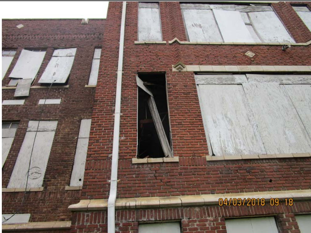
Exterior brick distress - cracking.
