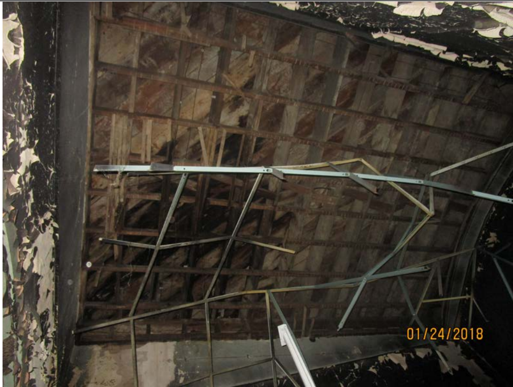
Wood floor framing deteriorated.
