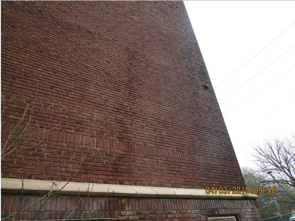
Exterior brick distress – water staining.
