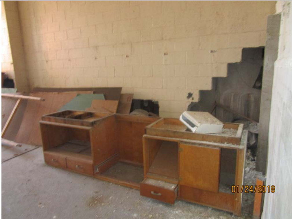
Interior CMU block wall damaged.
