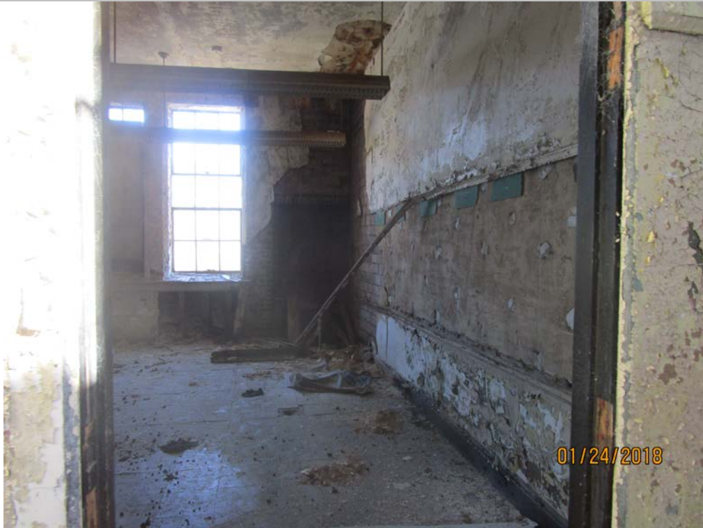
Roof system of left and right wing additions covered with plaster – further evaluation needed.
