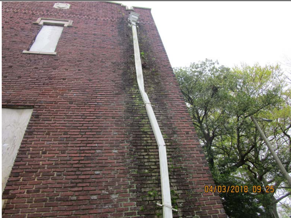
Exterior brick distress – water staining.
