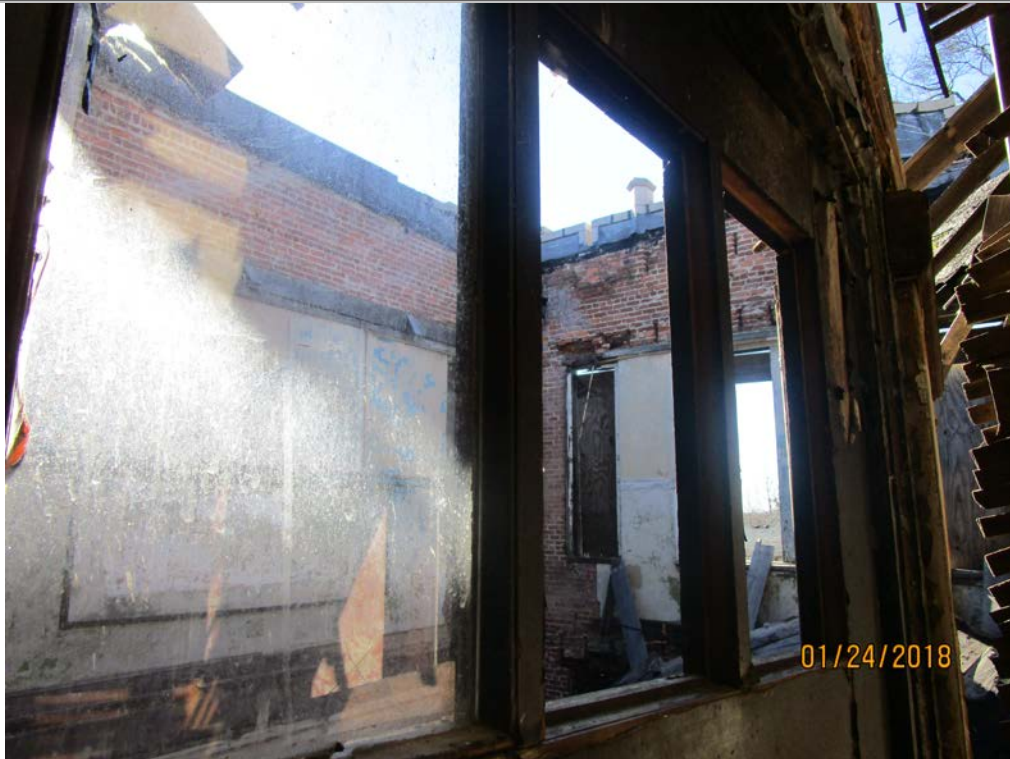
Roof framing collapsed.
