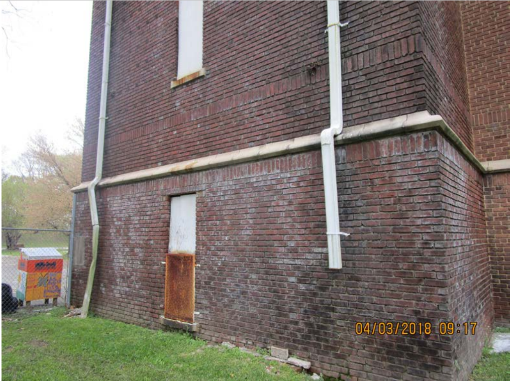
Exterior brick distress – water staining.
