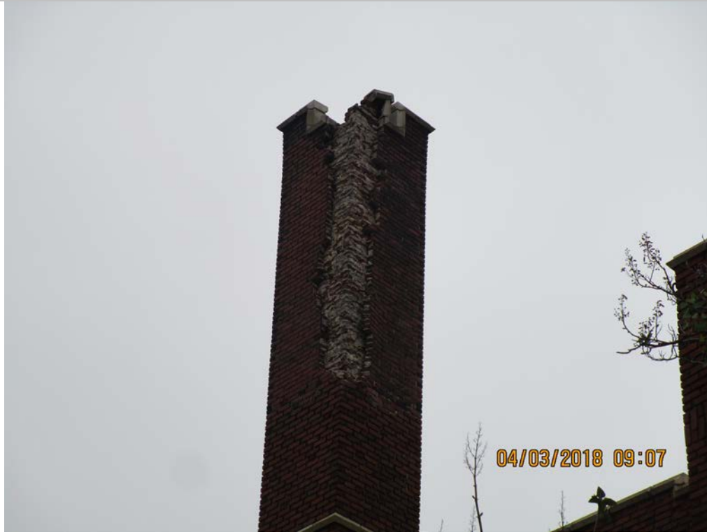
Exterior brick distress – cracking and collapse at top of boiler chimney.
